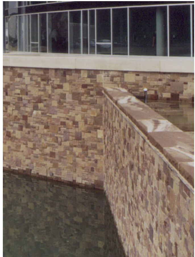
FIGURE 2.3: Ashlar sandstone veneer is used for its high aesthetic quality and cost-effectiveness at the Automated Transportation Management System Headquarters in Indianapolis
